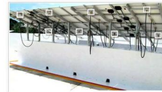
Figure 3. Location of the surface temperature sensors installed under the PV modules
