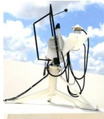
Figure 5. Image of the solar radiation station showing the tracking system and the set of radiation sensors installed.
