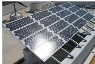
Figure 1. Photovoltaic energy generator comprising four sub-arrays of four PV modules each
