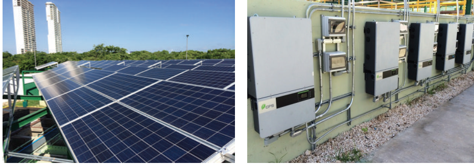
FIGURE 13: PV facilities of JAPAY in Merida city.
